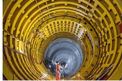
There are two of these 3 km long tunnels and two of the water intake heads will be fitted to each of them, sucking in 67 cubic metres of water and marine life per second.
